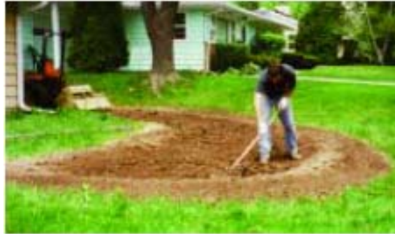
On a gentle slope, soil from digging out the garden can be used to create the berm. This rain garden is 4 inches deep.
